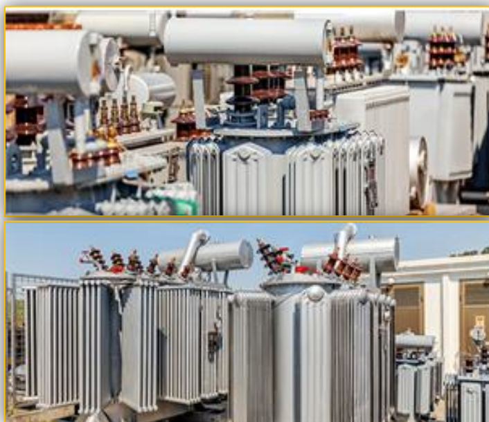
Figure 1. Pitch of 10-20 kW and 35 kW transformers operating in mining, [1], [8] to [10]
