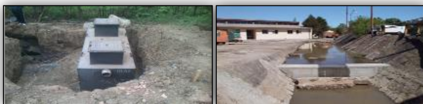
Figure 2. Installation of a separator for the treatment of oily waste water from car workshops and the new washing
